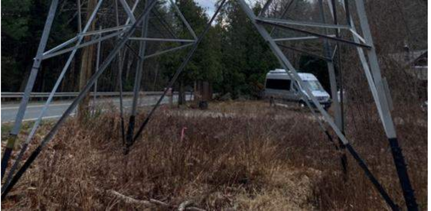
Photo #5: View of existing Structure 407 located within ORW BVW PE-W2A, B-407 is proposed approximately 19 feet northwest of the existing structure. Temporary construction matting in BVW is required in order to create a work envelope for the work. Facing south.
