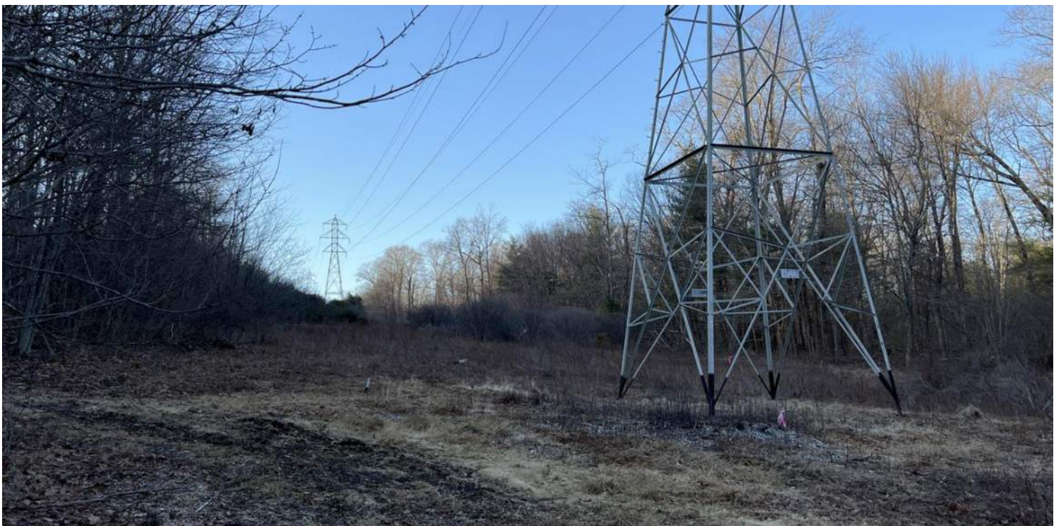
Photo #2: View of existing Structure 396 and ORW BVW PE-W6 (Str 395 in background). Temporary construction matting in ORW BVWs including PE-W6 is required in order to access B-390 located in upland. Facing southeast.
