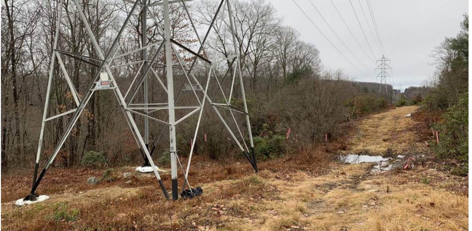
Photo #3: View of existing Structure 398 and ORW BVW PE-W8 (Str 397 in background). Temporary construction matting in ORW BVWs including PE-W8 is required in order to access B-377 located in upland. Facing southeast.
